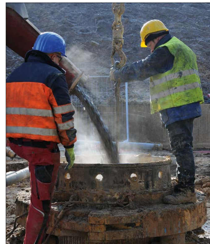
Eighty foundation piles are currently being driven into the ground to create the retaining walls of the GSI facilities. (Image credit: G Otto/GSI.)
